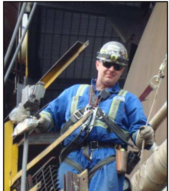
And Christian Brideau of Horton CB&I checks all his gear as he prepares to reinstall the deck and railings on level 6.5 of the Burner.
